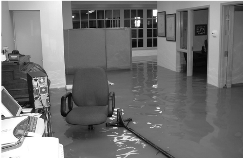
Flooded Allan & Stults office.
